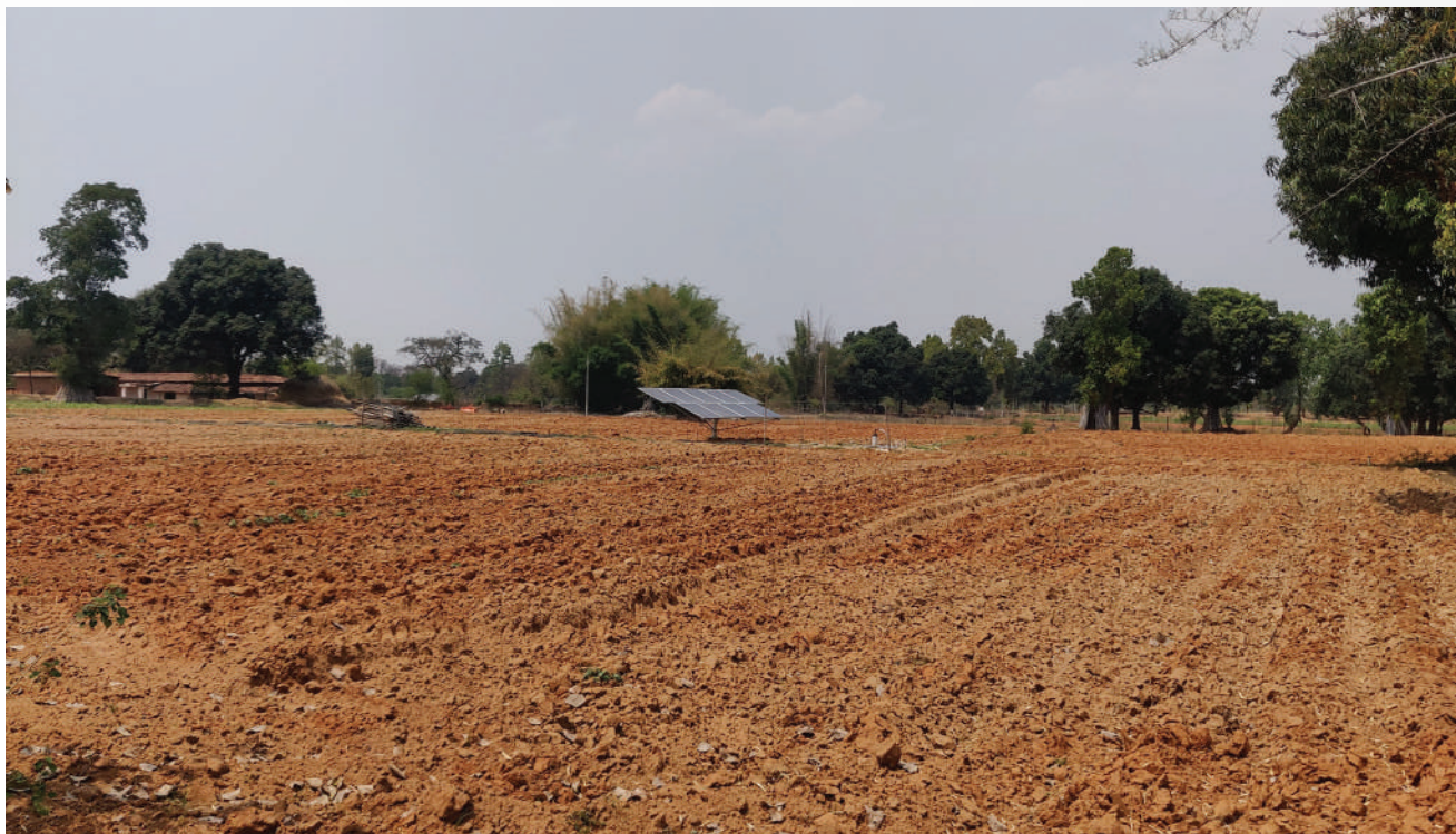
A solar pump installed for irrigation subsidised by the Chhattisgarh Saur Sujala Yojana. Photo Credit: Arpita Victor
