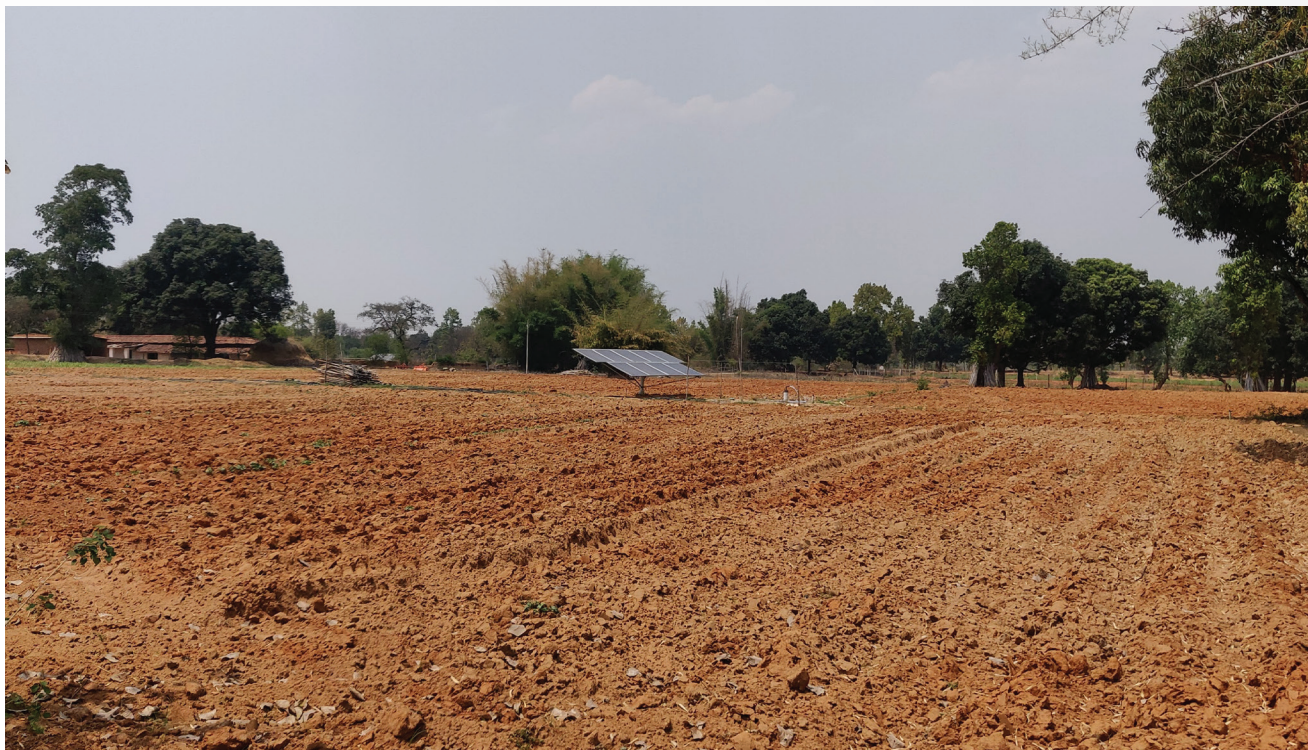
A solar pump installed for irrigation subsidised by the Chhattisgarh Saur Sujala Yojana. Photo Credit: Arpita Victor
